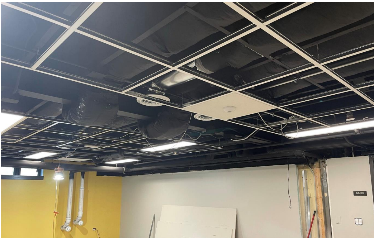
The ceiling grid in the sewing room is split into 3 "clouds", allowing for installation of acoustical tiles without lowering the ceiling to due to existing plumbing and structural components.
