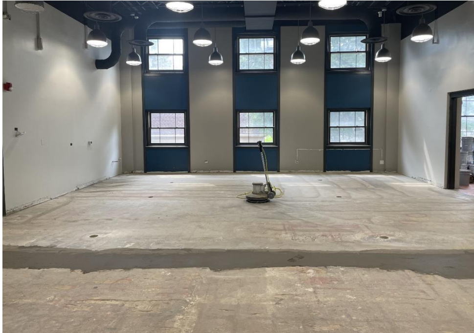
Before the new flooring was put in place, prep work included removing the old adhesive, filling any imperfections in the subfloor and sanding everything smooth. In the main makerspace area, there is a joint where the concrete floor mates with the wood subfloor. This picture shows the work on the transition between the two surfaces to level it and make it as stable.
