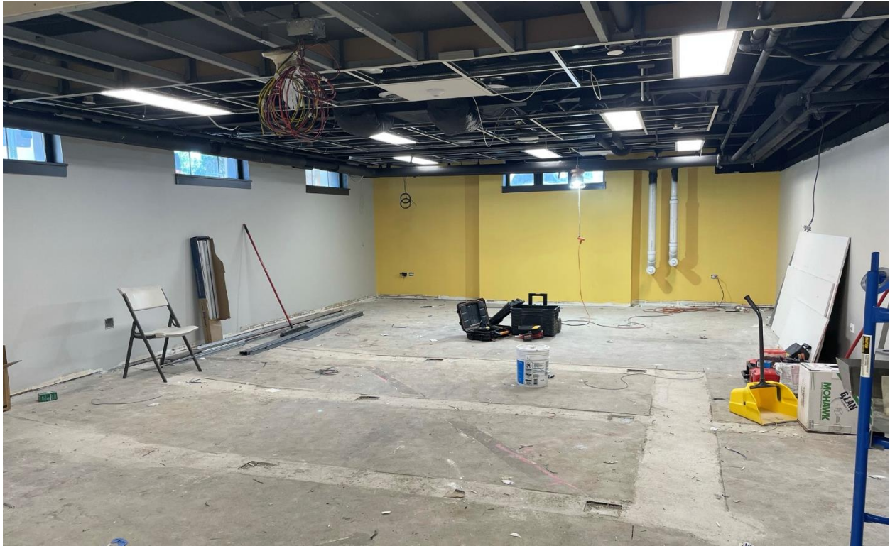
The sewing room ceiling awaits inspection before installation of ceiling tiles. With the electrical work in the floor completed, tile work can commence.
