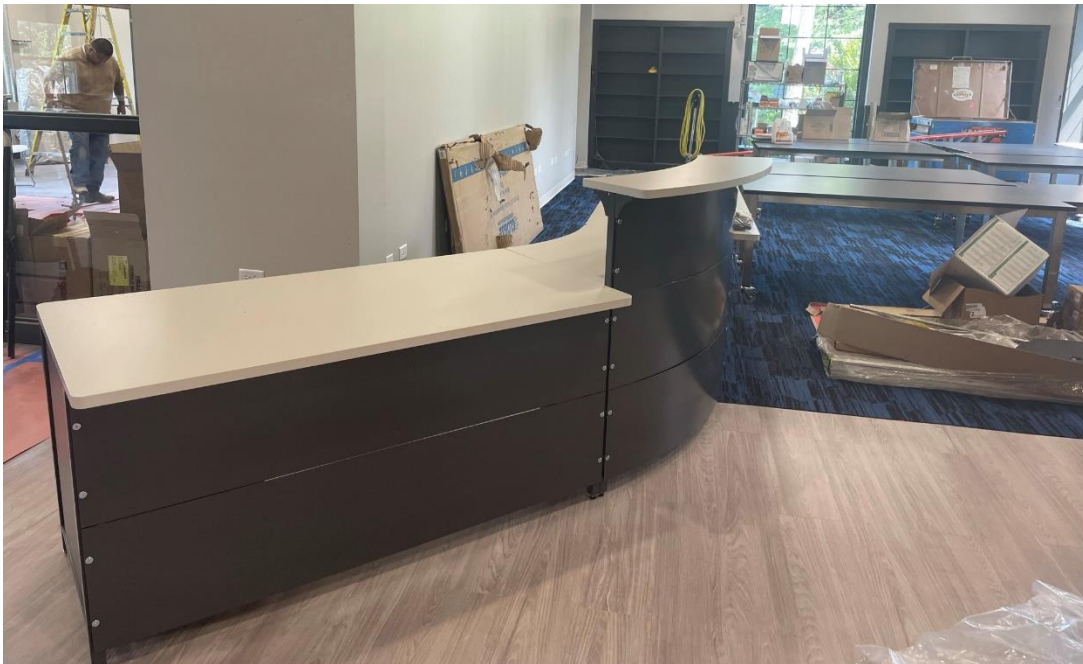
The new public service desk has been delivered and assembled. This desk will be large enough to accommodate two staff members and will be located near the entrance, one of the first things a customer will see when entering the space.
