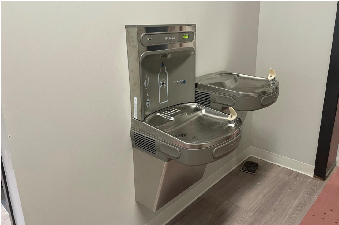
New water fountains and water bottle filling station are installed in the main floor hallway.
