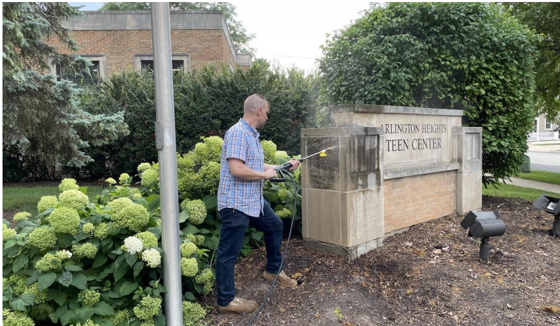
In preparation for the installation of the new sign inset, Eric Massingill and Dan Teuber pressure washed the concrete and brick monument.
