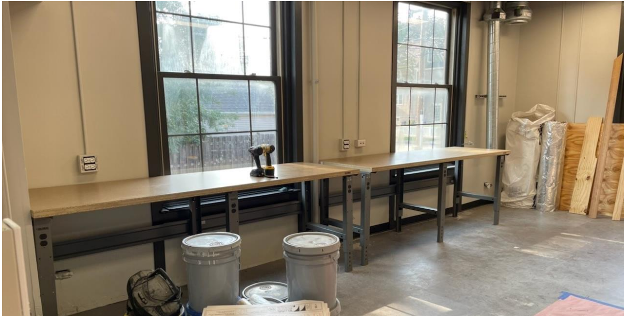
The Industrial Tools room is taking shape with the installation of the worktables. These tables will be home for one of the laser cutters, a CNC machine and vinyl cutters. Getting these in place allows us to plumb the ventilation required by the laser cutters.
