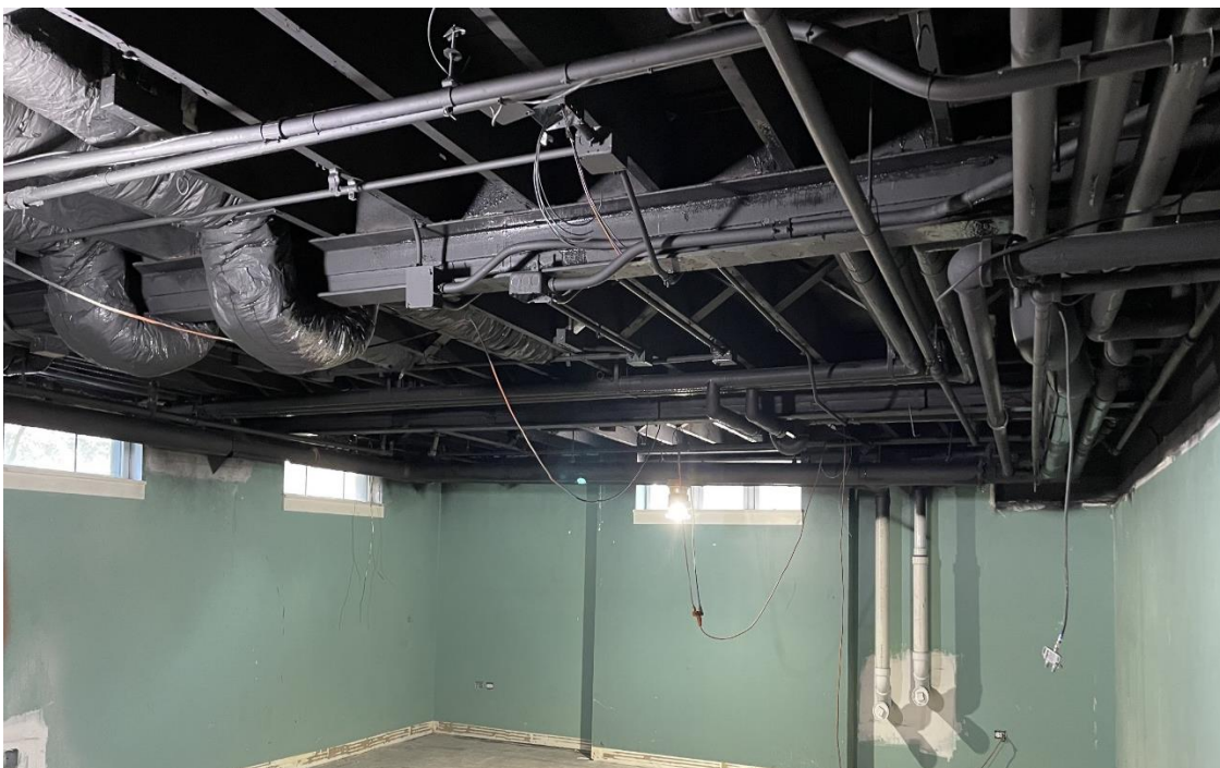
The sewing room ceiling received a coat of black paint before the installation of the grid of ceiling tile "clouds", which will provide acoustical absorption and provide a place to mount the new LED lighting. The ceiling in this room was re-engineered in the field to accommodate structure and utilities that would have otherwise reduced the height significantly.
