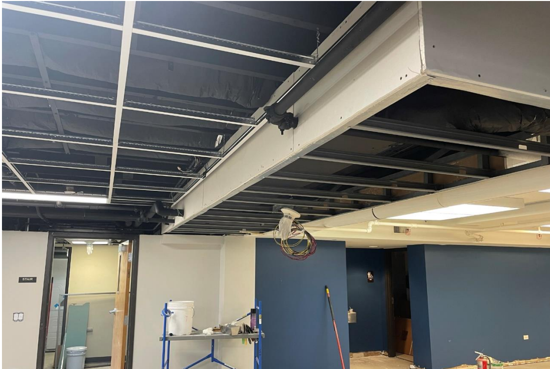
Ceiling grid and soffit are installed in the sewing room around existing plumbing and conduit.
