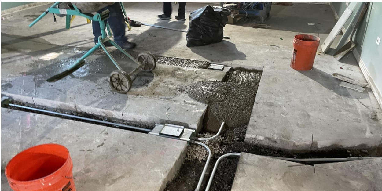
The electrical work in the sewing room floor included saw cutting the concrete floor and installing floor outlets. New concrete has been poured after conduit and outlet boxes have been installed and inspected. These outlets will provide power to the individual sewing tables.
