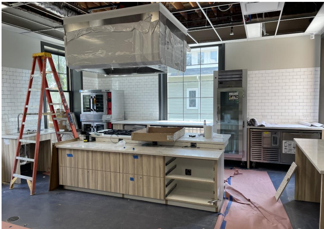
The kitchen nears completion after the installation of appliances. Ceiling grid tiles will be installed after electrical and sprinkler inspections are completed.
