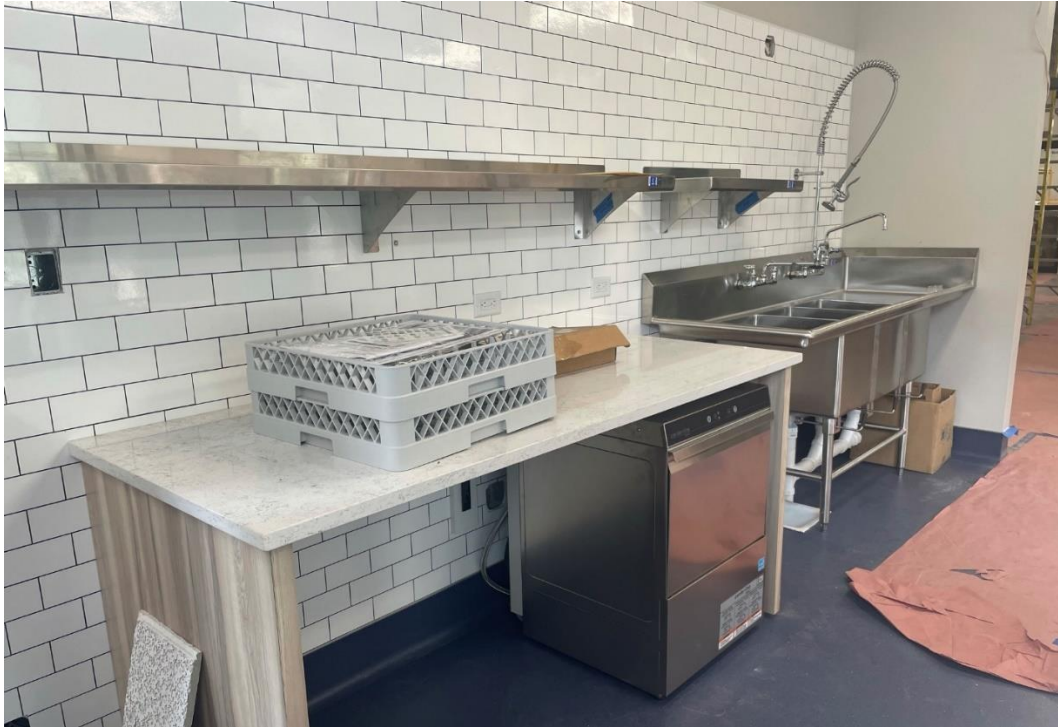
Plumbers have been on-site installing the kitchen equipment. The three-compartment sink is nearly ready for use, as well as the handwashing sinks, prep sink and dishwasher.
