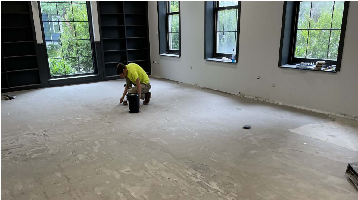
Much of the plywood subfloor throughout the main floor suffered some damage during demolition. With the help of our staff securing the subfloor, the flooring contractor was able to fill and level the surface to prepare for carpeting.
