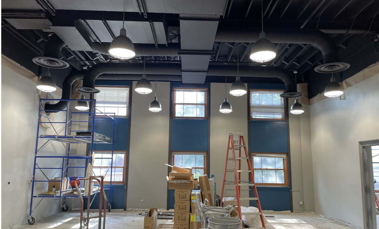
Installation of the lighting is complete on the main floor. The pendant lighting shown above is the result of acceptance of the lighting upgrade package add-on.
