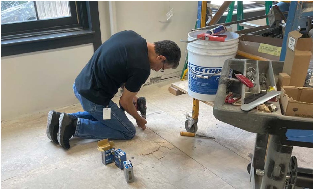
Facilities staff, Jim Hawkins, secures the subfloor to remove any movement or squeaks in preparation for new floor covering.
