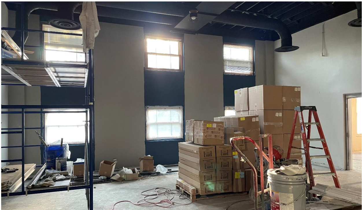
Paint applied in the main makerspace area. In the foreground, lighting fixtures await installation.
