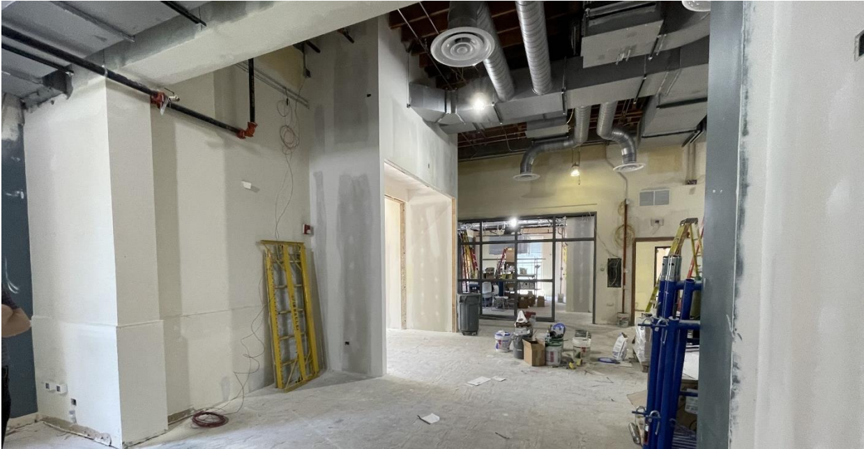
Drywall taping and finishing is complete throughout the building and walls are ready for primer and paint.
