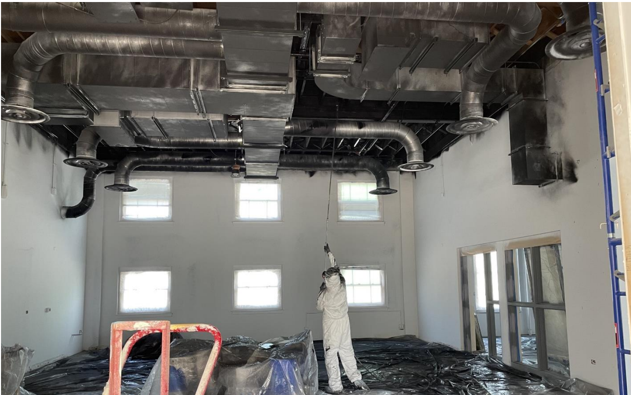
Painters apply black paint to the ceiling and ducting in the main makerspace area (flex 1).
