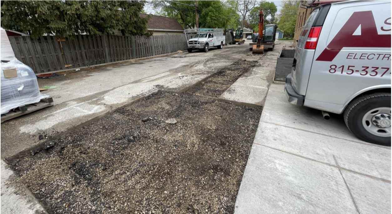
A strip of the parking lot was excavated last week to make way for our new hook-ups to the village sewer. The really impressive part is that it was completed in a day to minimize street closures.
