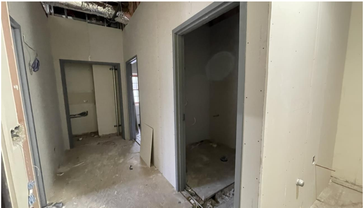
Framing and drywall are complete throughout the building. Contractors are currently preparing the surfaces for paint by filling holes and taping seams.
