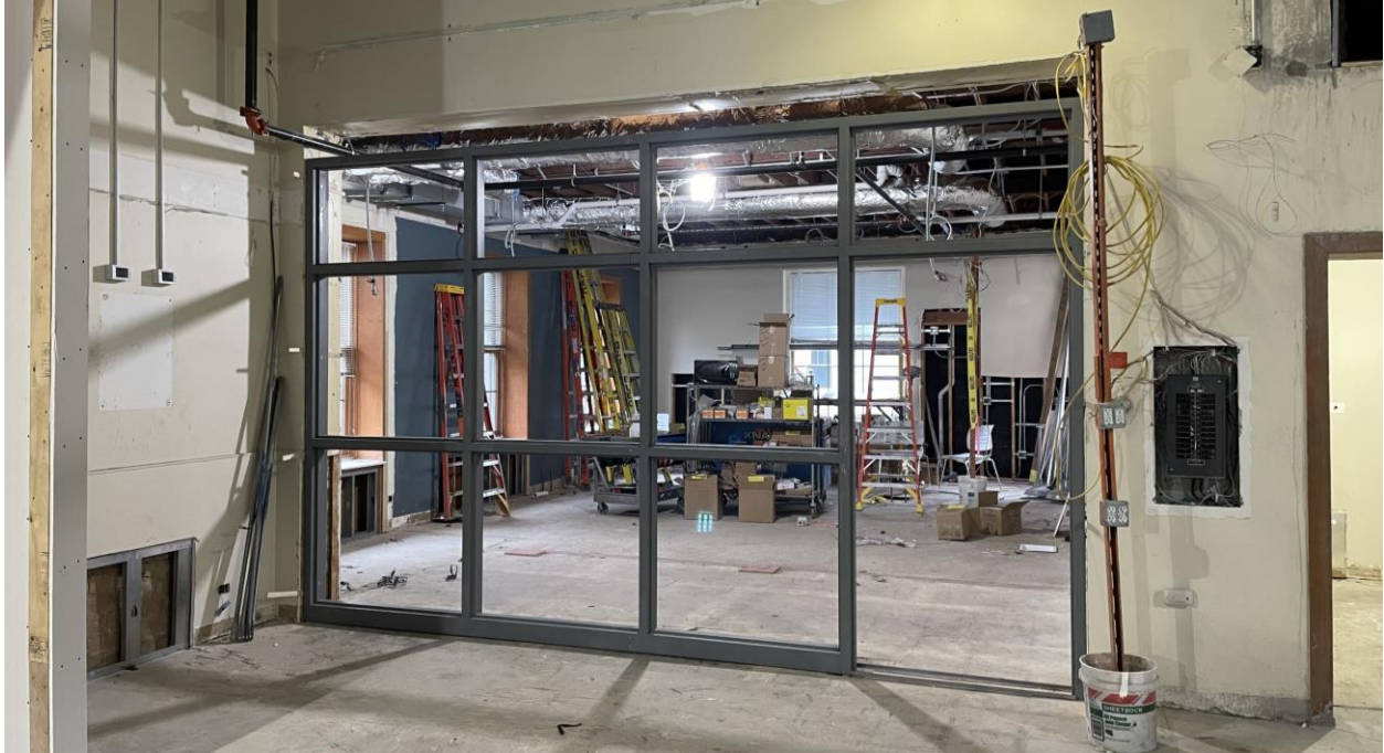
The new metal framing for the kitchen entrance has been installed and looks great. This frame (just like the industrial tools room) will be filled with glass windows and doors so makerspace users can get a look into the kitchen while still keeping some of the clanking dishes, whirring mixers, and delicious smells trapped inside.
