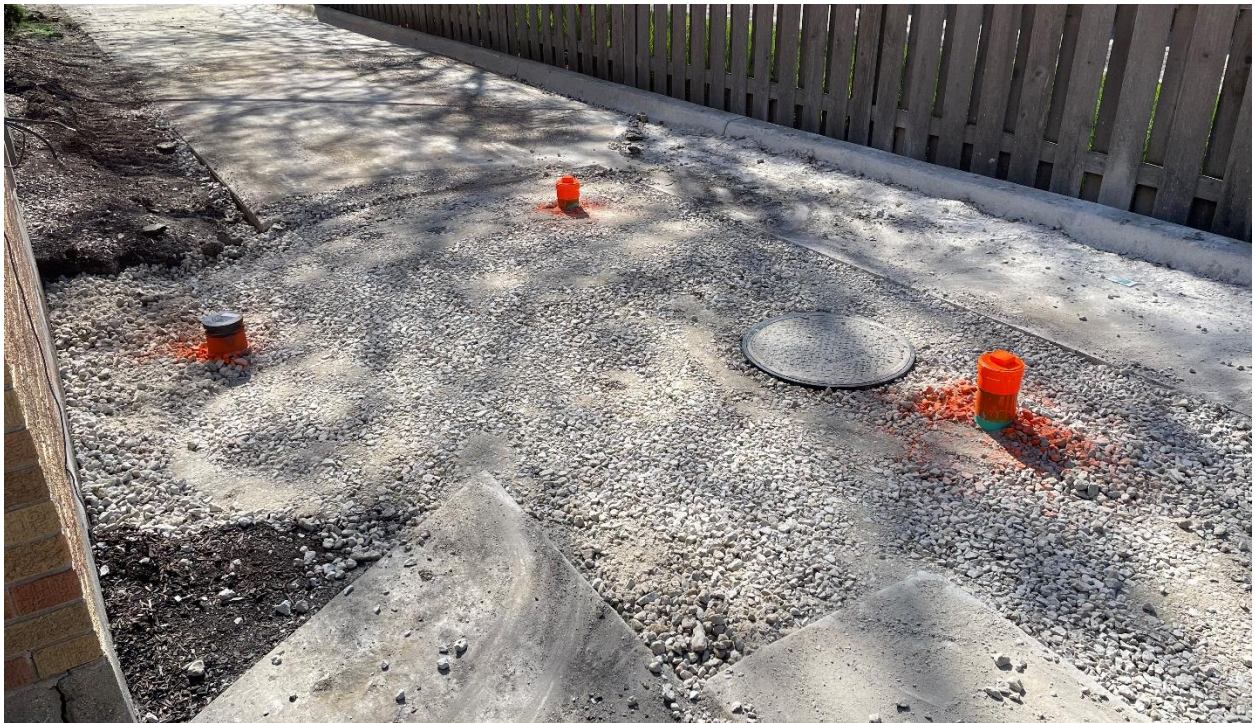
The new commercial kitchen grease trap has been installed under the driveway on the south side of the building.
