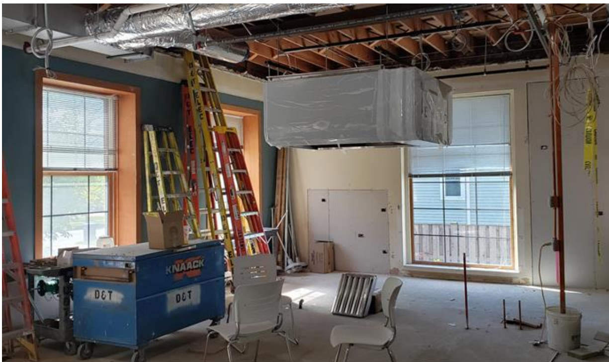
The kitchen hood, paid for by the AHML Foundation, has been hung in place.
