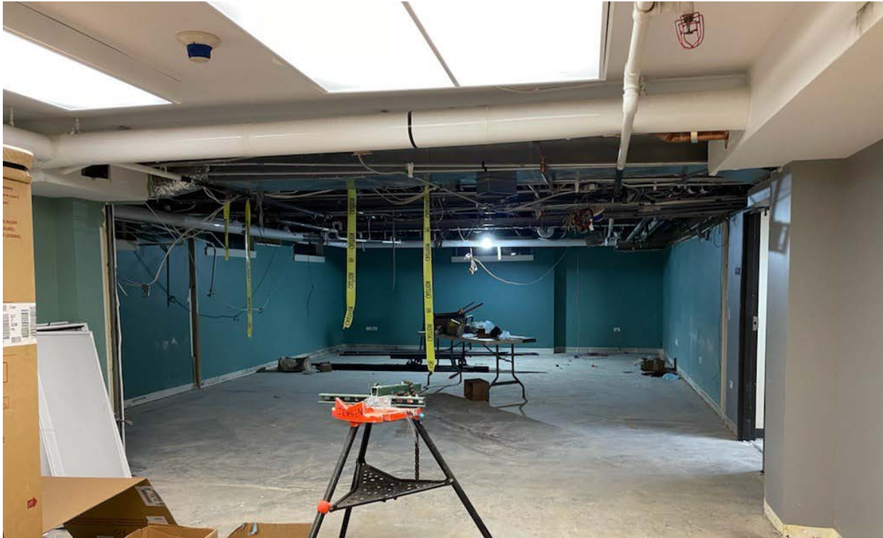
Demolition of the walls and ceiling for the new sewing room is complete.
