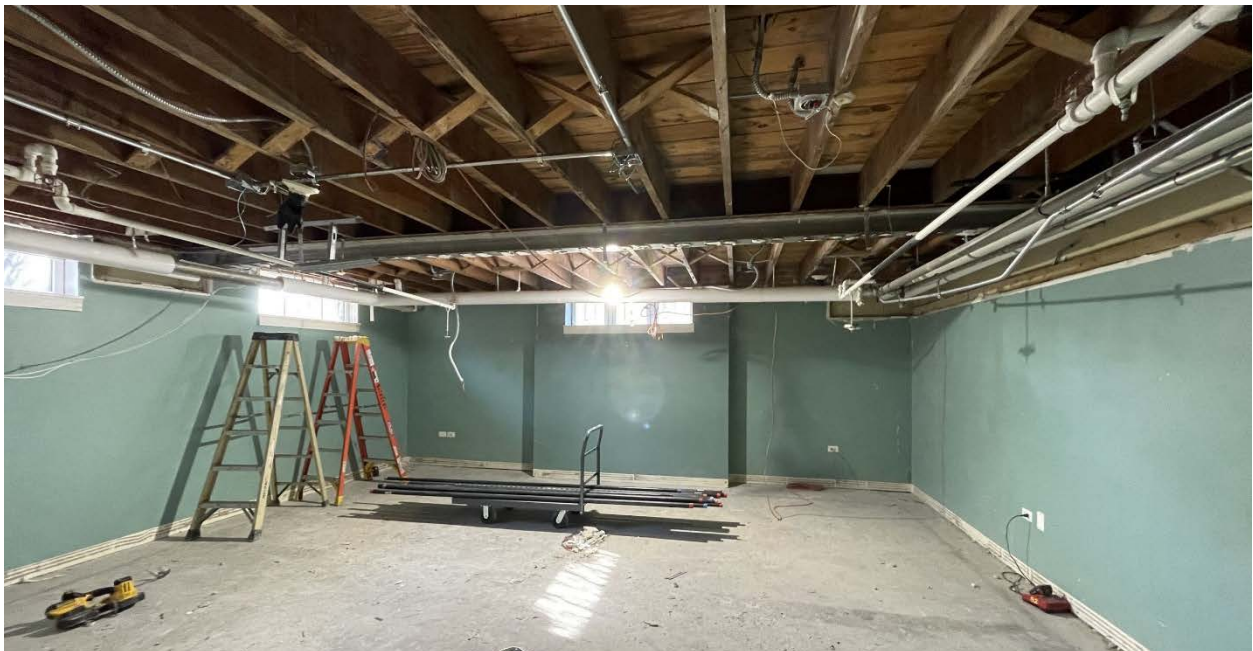
Plumbing for the first-floor restrooms, and commercial kitchen, including the 3-compartment sink, vegetable sink and floor drains has been installed in the basement ceiling. Installation of the grease trap and outdoor plumbing is underway.
