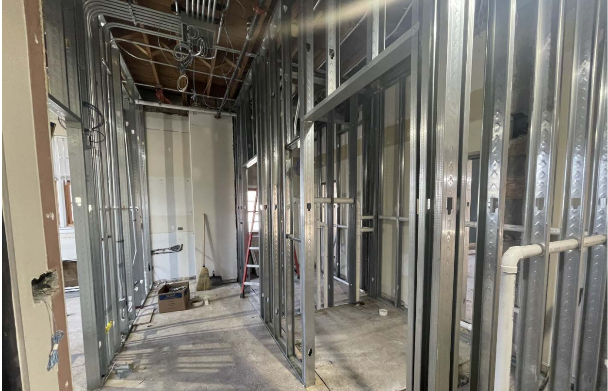
Reconfigured first-floor restroom area includes a new hallway outside the assistant manager's office, relocation of the restroom doors, and a janitors' closet at the end of the hallway.
